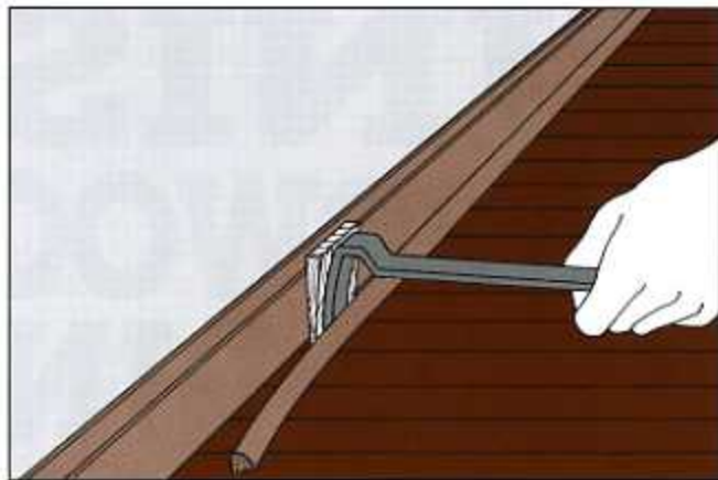
Fig. 1. Before sanding an old floor remove the base shoe. Use a wood wedge behind the pry bar to protect the baseboard from damage by the bar.
